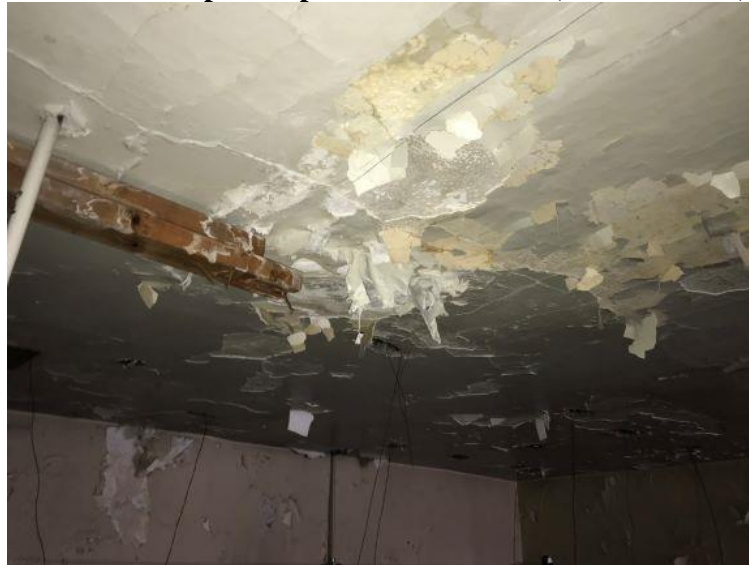
Mechanical Dept. – Superintendent Office (water intrusion)
