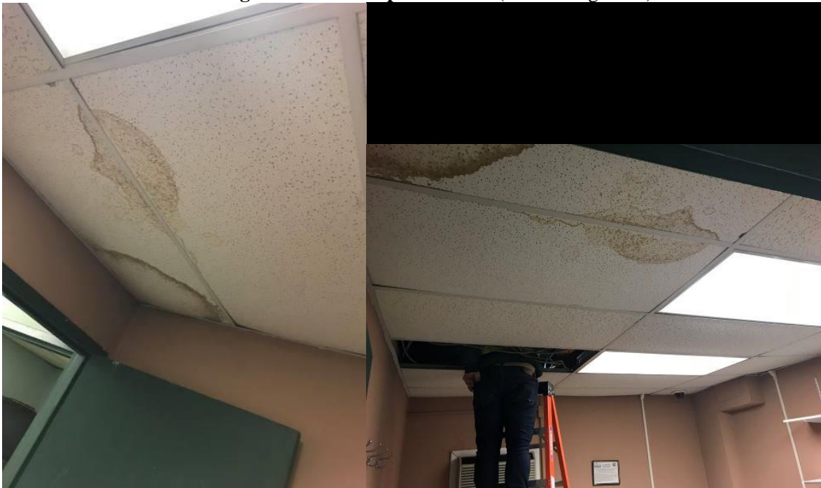
Training Room 8A-Computer Room (microbial growth)
