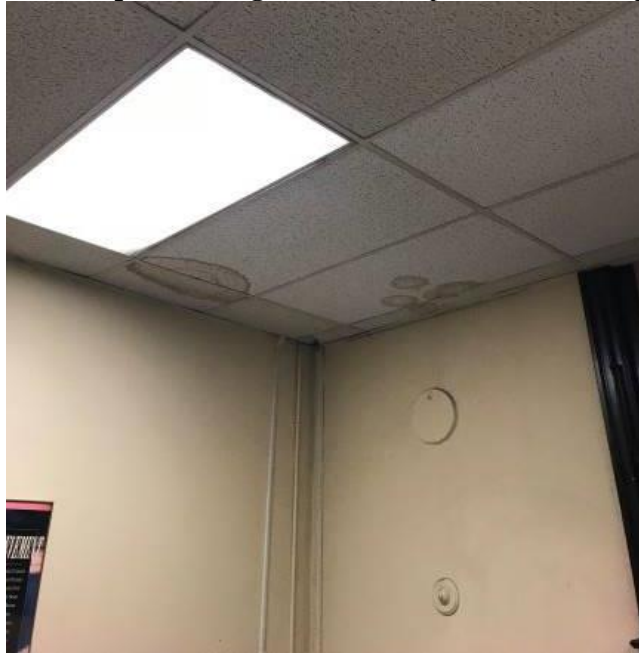
Mechanical Dept. – Manager Office (suspected microbial growth)
