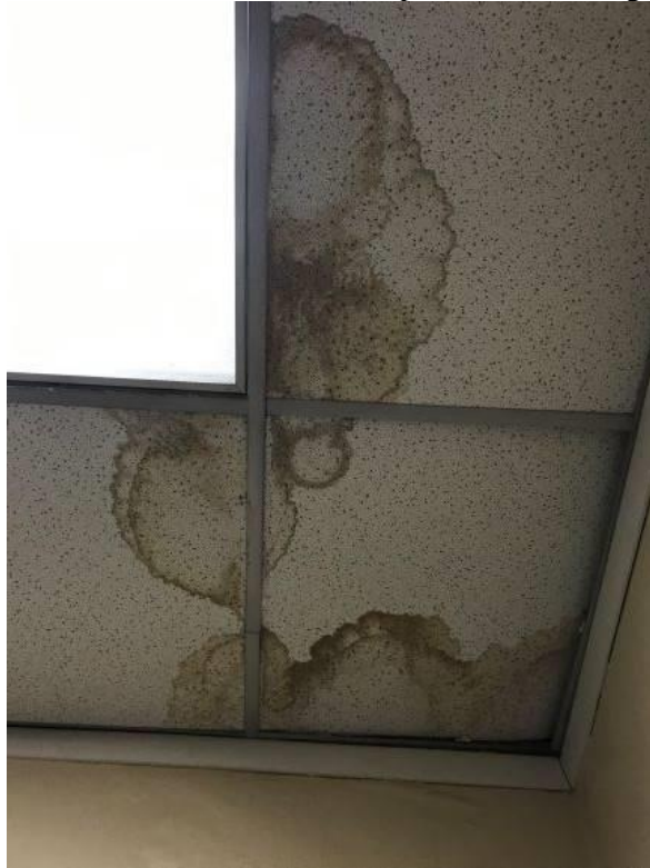
TCU Break Room/Bathroom (suspected microbial growth)
