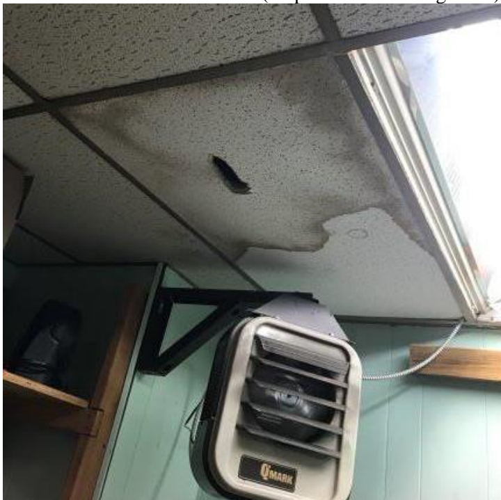
Railman for Children Office (suspected microbial growth)
